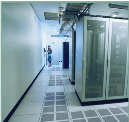
Precision Air Conditioning
